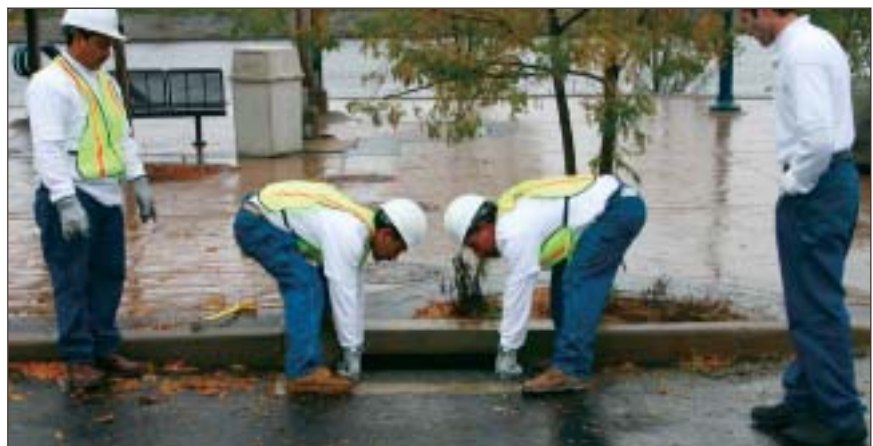
...placed the filter, and put the grate back in place, completing the installation.
